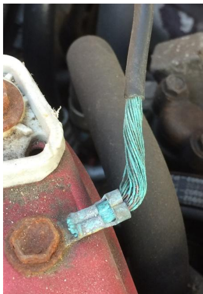
Corrosion on grounding wire
